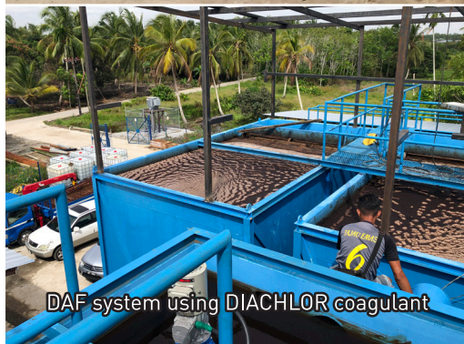
Coagulant dosing system
